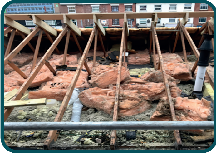
What was found when the tiles were stripped - an insulated loft – really?
