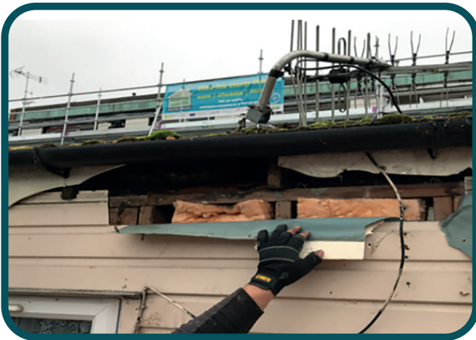
Original insulation installation within the timber frame panel – significant thermal by-pass
