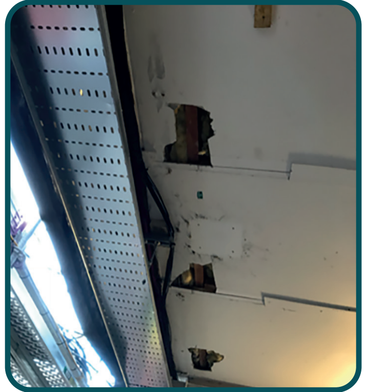
An undercroft soffit, below a kitchen - no insulation when built.
